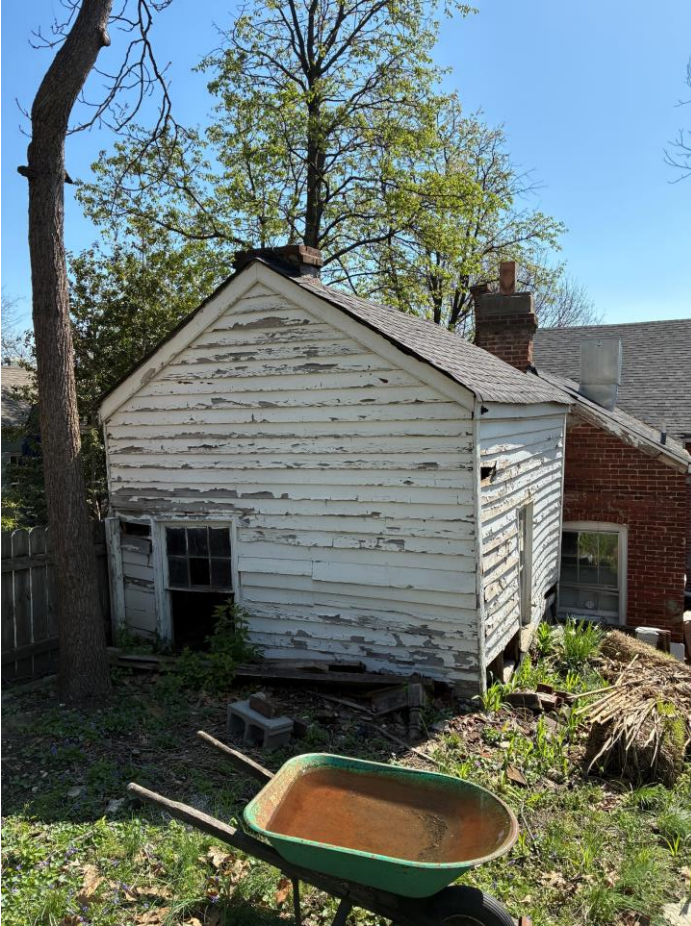
HISTORICAL/ARCHITECTURAL ASSESSMENT 519 S. Main Street Rear Frame Outbuilding; South Main Street Preservation District
