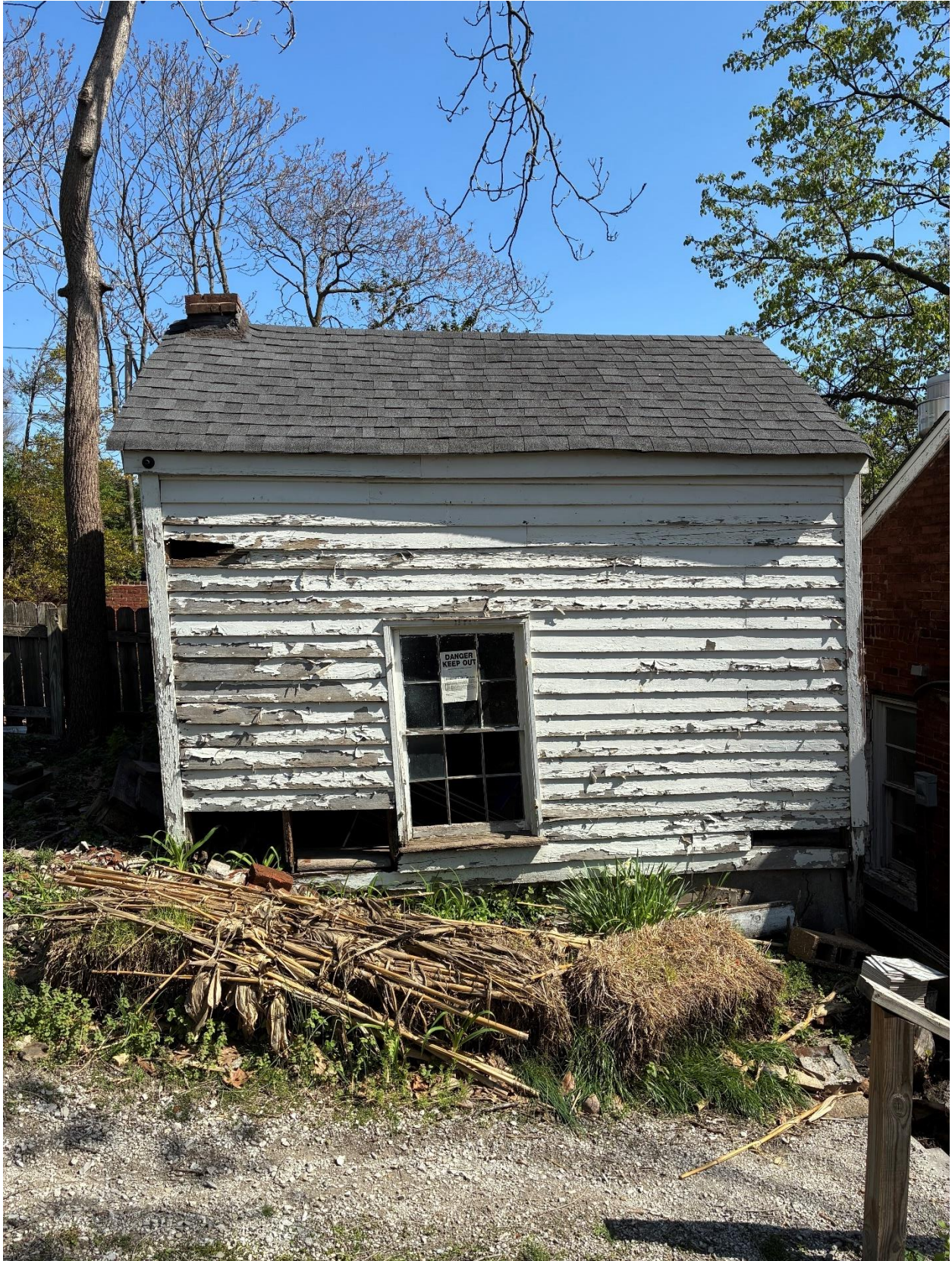
Photo 2: View facing north. Historic 6/6 double-hung wooden sash intact, but missing lights
