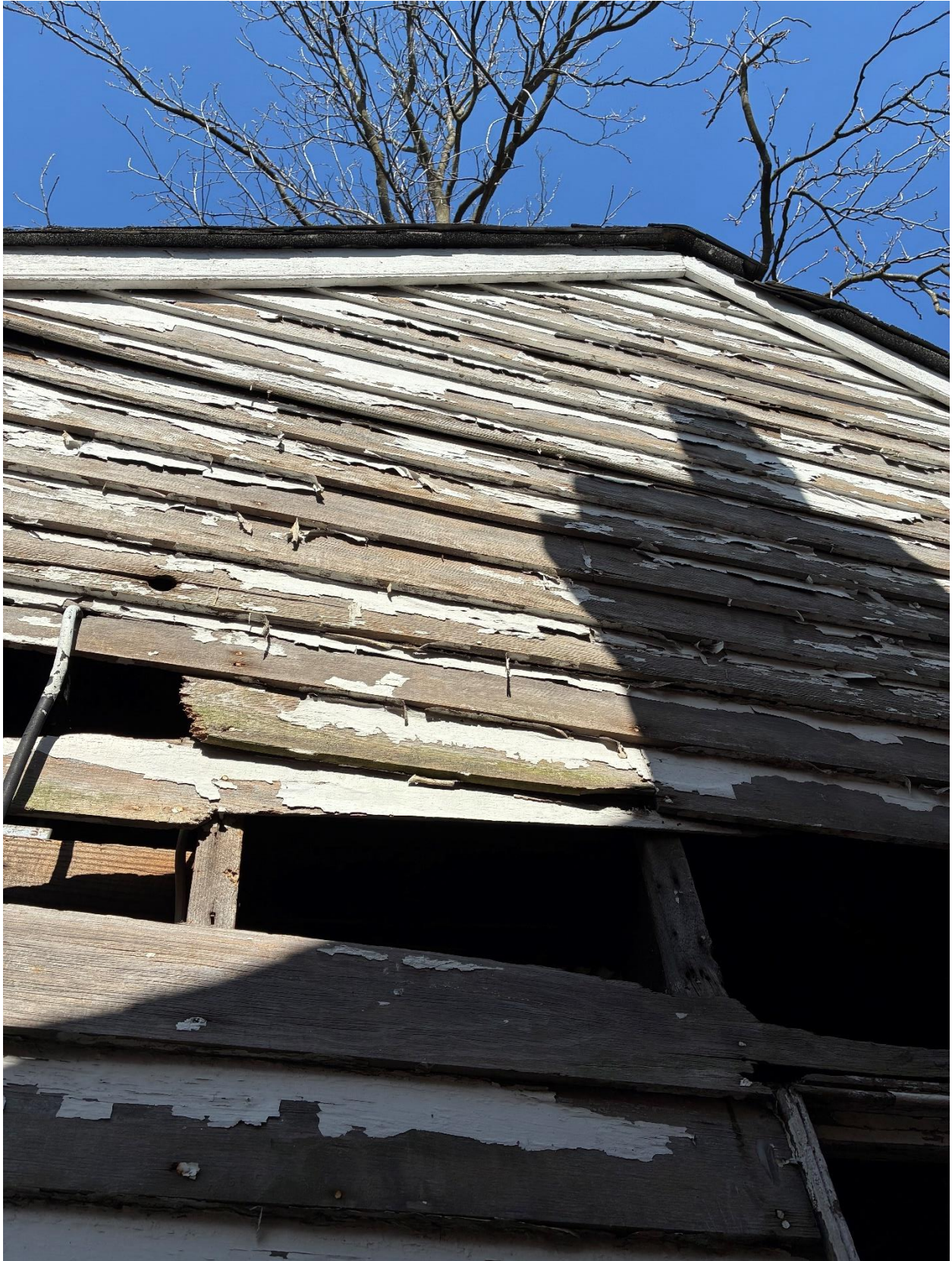
Photo 7: Condition lap siding
