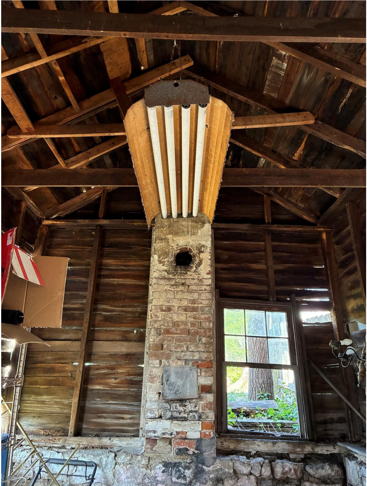
Photo 6: Interior facing west. Ad hoc reinforced structure. Chimney with stove pipe aperatures
