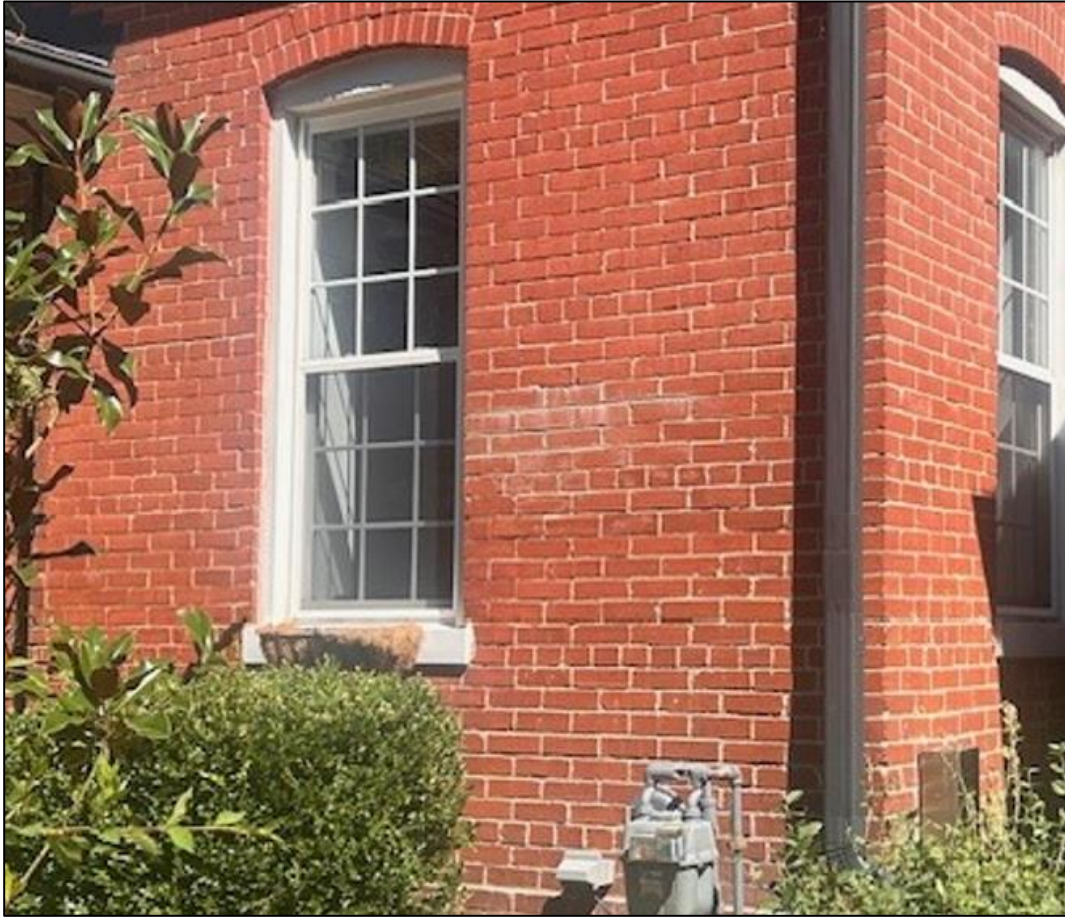
Figure 3: Brick damage example 2.
