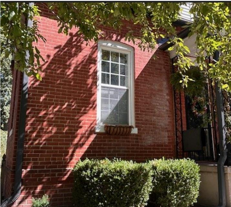
Figure 2: Brick damage example.
