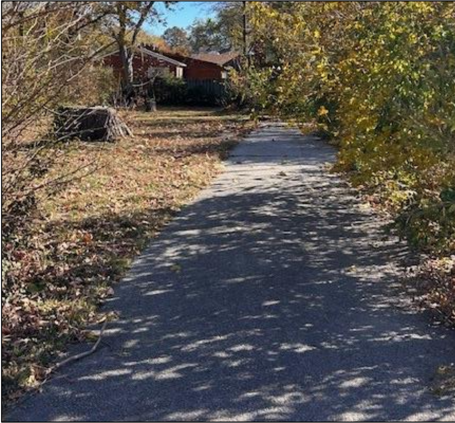
Figure 12: Driveway seen currently on the property to be repaved.
