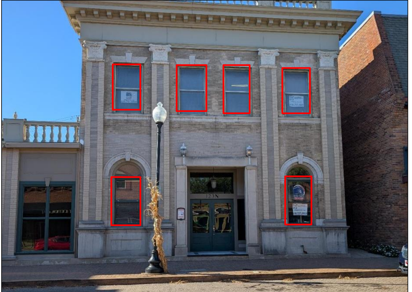
Figure 1: 123 North Main Street seen currently, showcasing the six subject windows for replacement.
