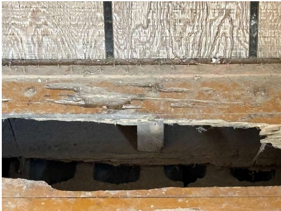
Deteriorated Sill plate
