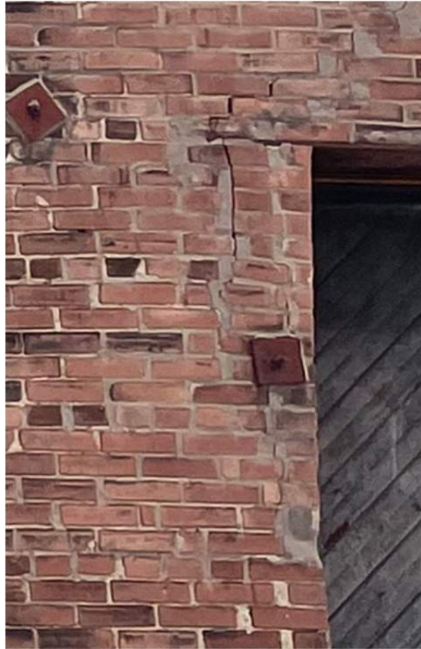
Image 25: South Building Wall Jamb Destabilization Example
