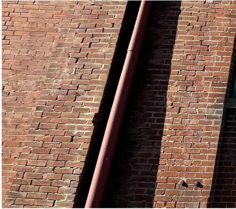
Image 22: Exterior Wythe Mortar Loss Example
