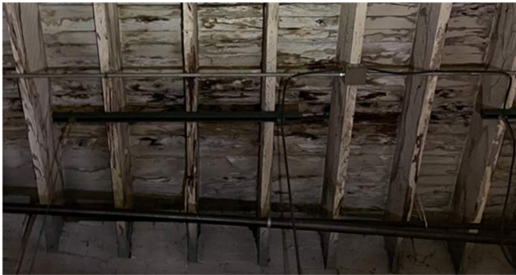
Image 16: South Building Second Floor Decking Water Infiltration Staining Example
