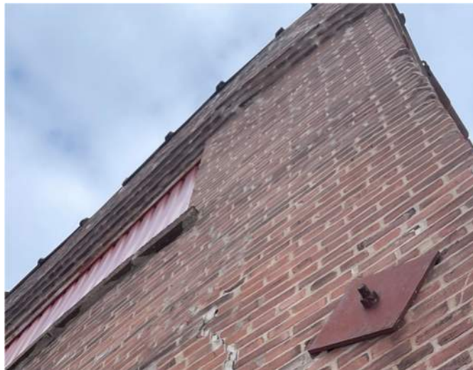
Image 24: South Building Parapet Bow and Wall Bow Example
