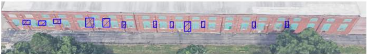
Image 23: Southern Exterior Masonry Areas of Mortar Loss
