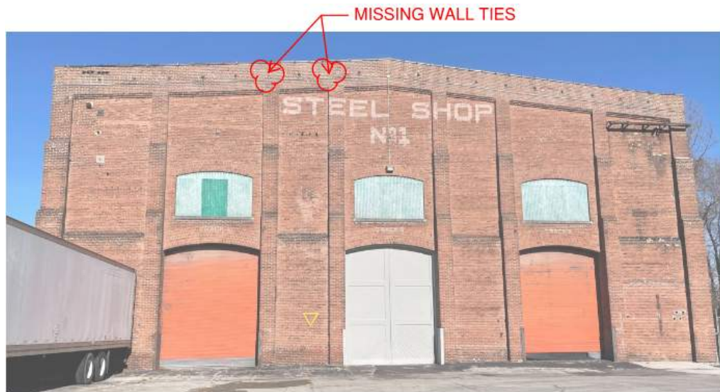
Image 17: Southern Wall Missing Roof Anchor Ties
