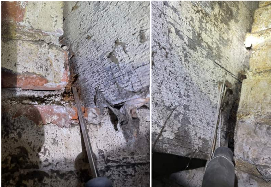
Image 18: South Building Second Floor Joist Bearing Rot Probe Examples
