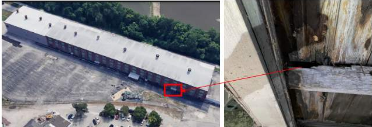
Image 13: Southern Building South-Western Shed Extension Roof Rot
