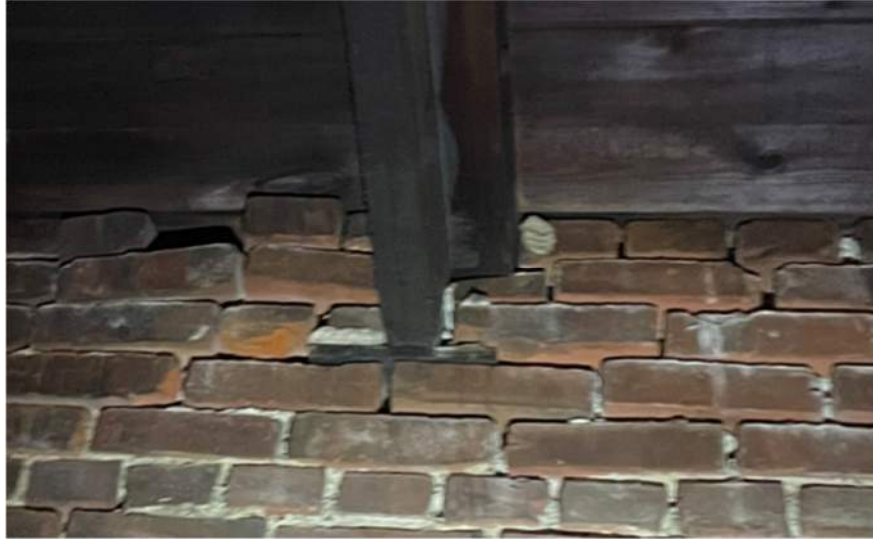
Image 14: South Building Roof Steel Channel Beam Bearing Wall Deterioration
