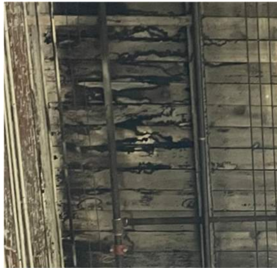
Image 11: South Building Roof Wood Deck Board Staining Example
