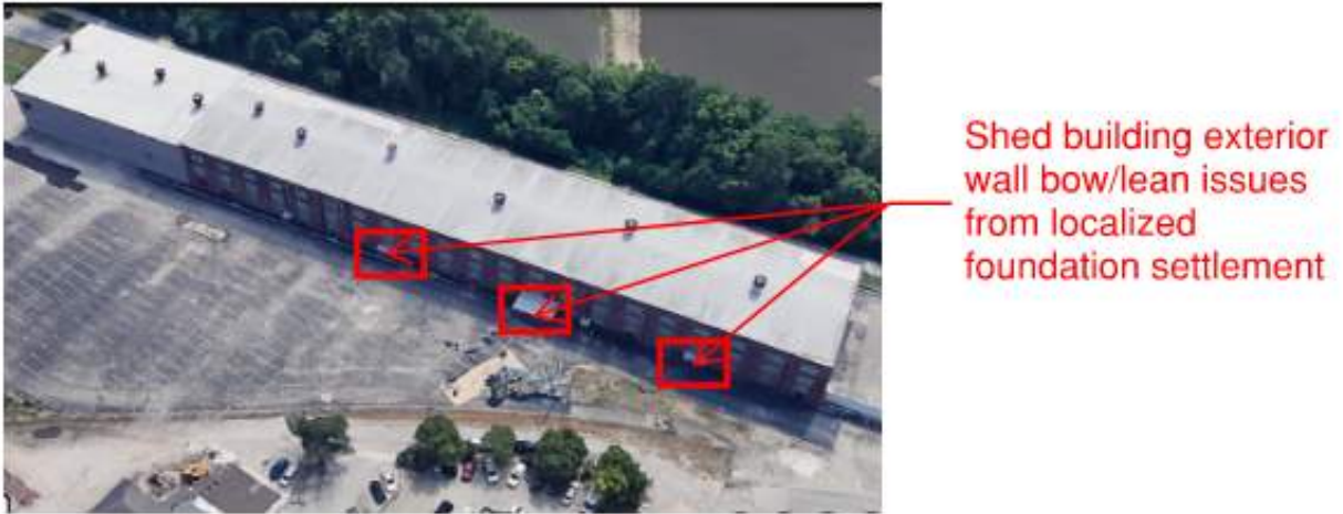
Image 14: Southern Building Shed Extension Locations of Observed Wall Destabilization
