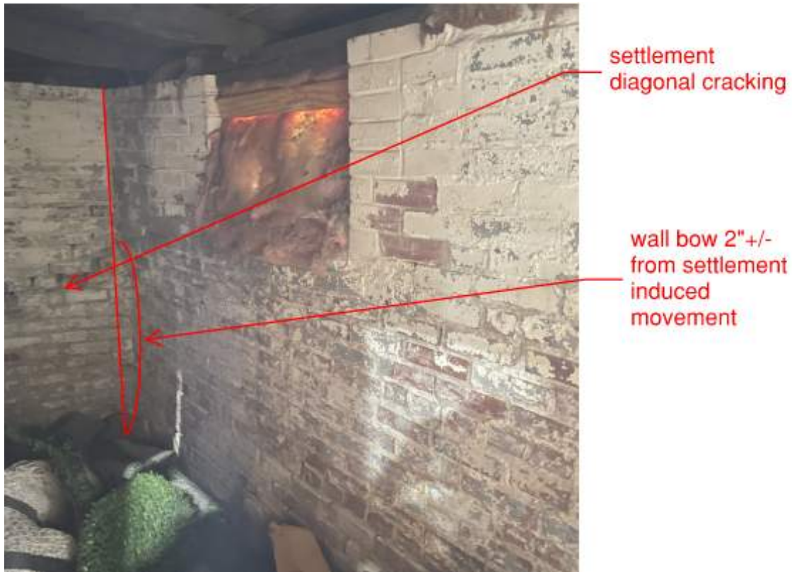
Image 16: Southern Building Shed Extension Movement Example
