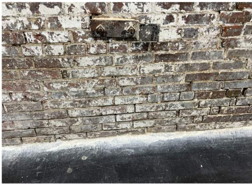
Image 18: Interior Wall Face Mortar Deterioration/Missing at Base of Wall
