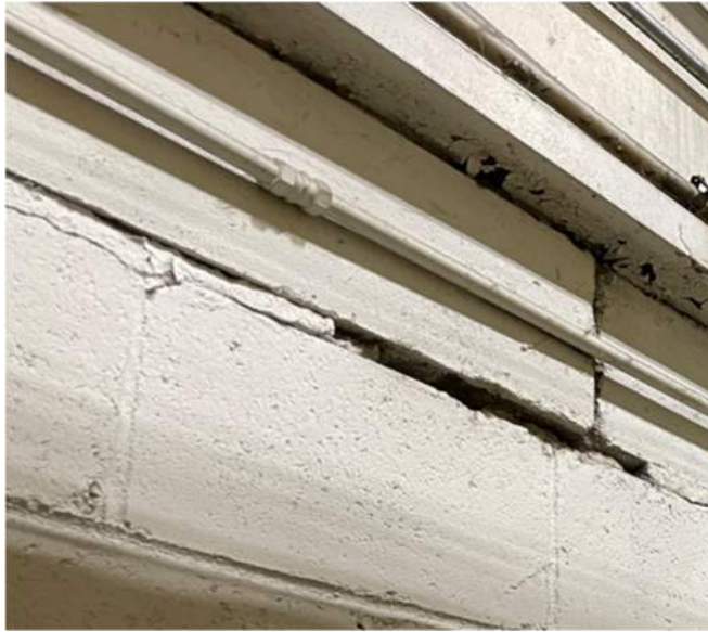
Image 26: North Building Perimeter CMU Wall Top Course Destabilization Example
