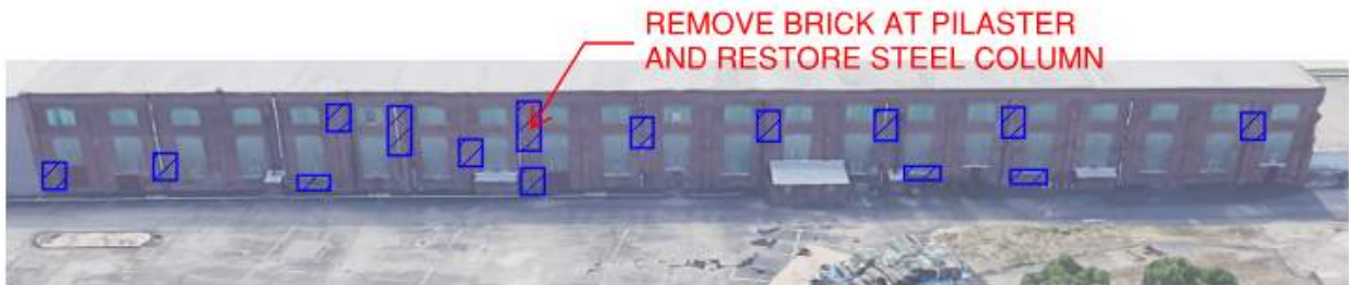
Image 24: Eastern Exterior Masonry Areas of Mortar Loss
