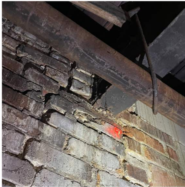
Image 15: South Building Roof Steel Girder Bearing Wall Deterioration with Bearing Plate Corrosion
