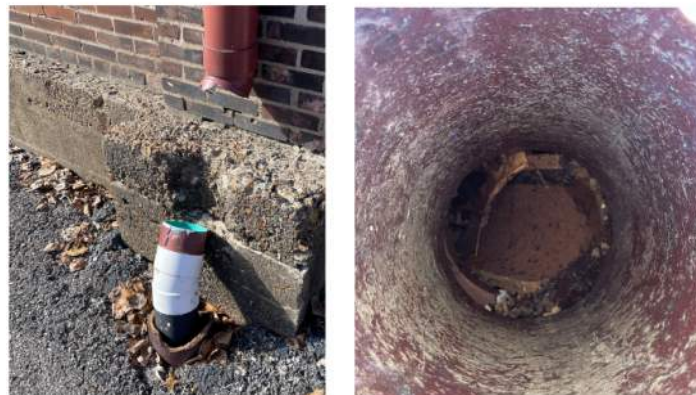
Image 21: Exterior Roof Drainage Pipe Damage and Terra Cotta Installation Observation
