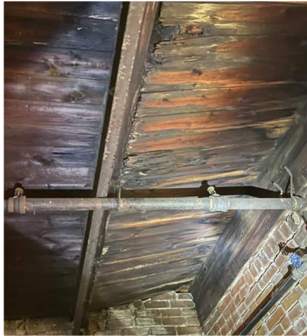
Image 12: South Building Roof Deck Rot Example
