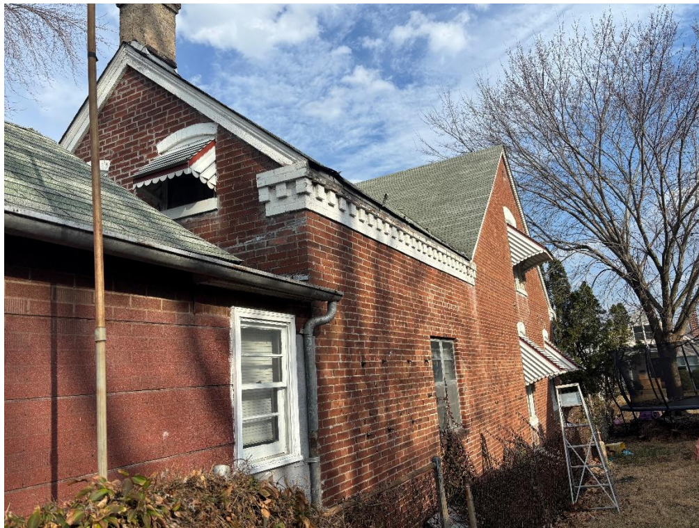
Existing Photo, Feb. 2026 – View of house from side yard looking east. Portion of home to be demolished shown a left of photos. Center shows likely masonry addition at rear of 1890 structure (furthest portion of photo to the right)
