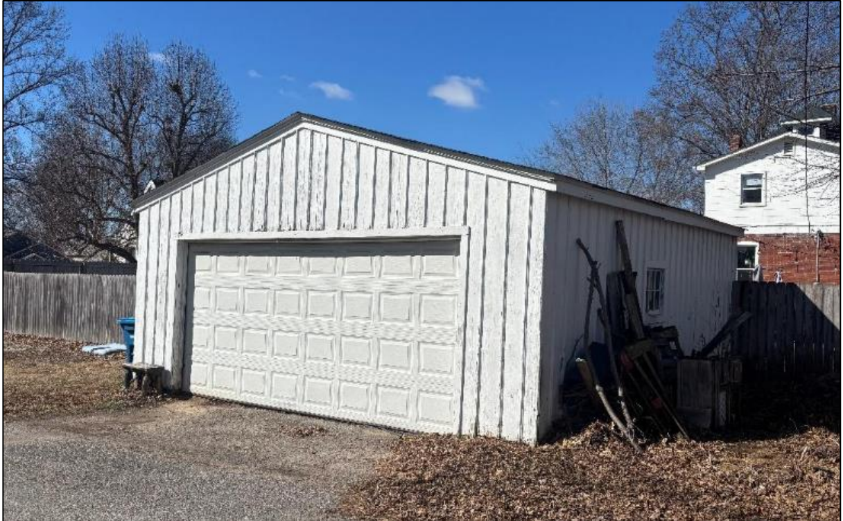
Figure 2: Subject structure seen from rear alley.
